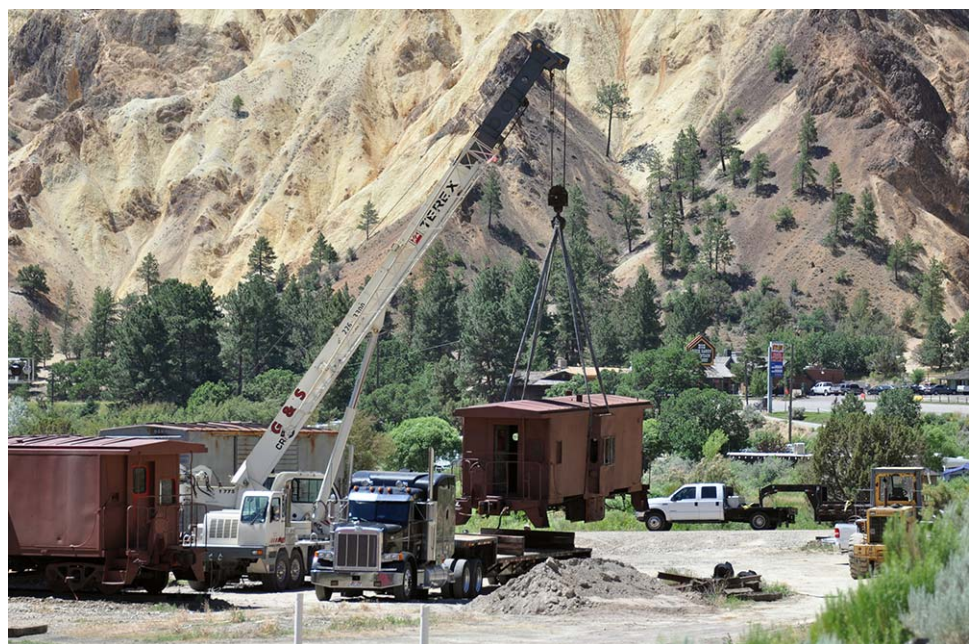
A crane puts a rail car into place at the Caboose Village Resort at Big Rock Candy Mountain. Photo courtesy of Sue Wood and Environetics.
