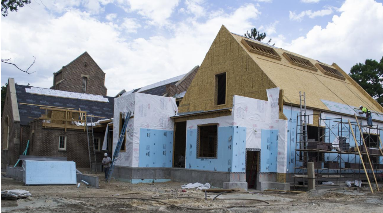
Renovation under construction designed by a historic preservation architect to have the addition blend in with the existing historic building. (Picture courtesy of Lori Wait)
